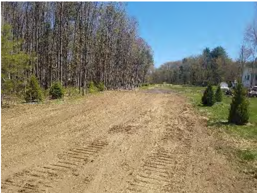
Fig 16: Restoration of access road from Nimble Hill road to Str. 107. Viewing northeast. (05-13-20).
