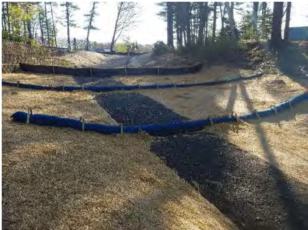
Fig 8: Finished restoration of slope from man hole to the salt marsh at Gundalow landing/east side of bay. Viewing east. (05-11-20).
