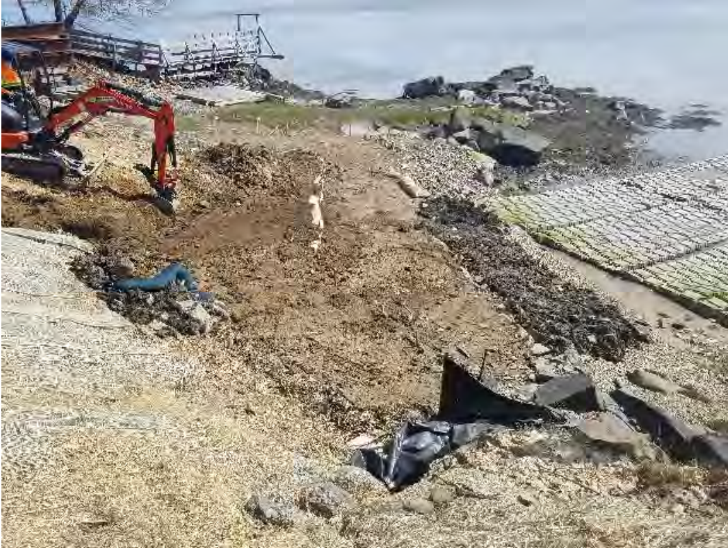
Fig 7: Salt marsh restoration underway at Getchell property/west side of the Bay. Viewing north. (05-08-20).
