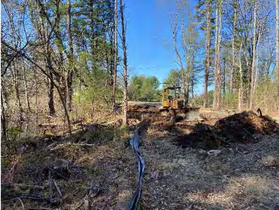
Fig 1: JCR beginning to relocate access road at Flynn pit to Str. 100. Viewing west. (05-07-20).
